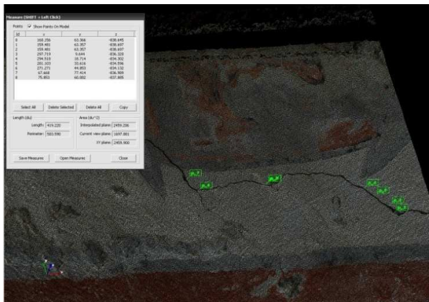
Figure 9a. Fissures measuring.
